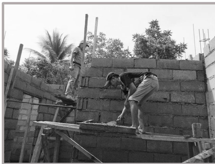
Figure 1. Hazard in workplace
